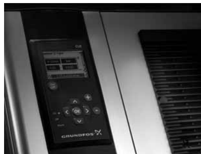
Fig. 25 Grundfos CUE control panel
