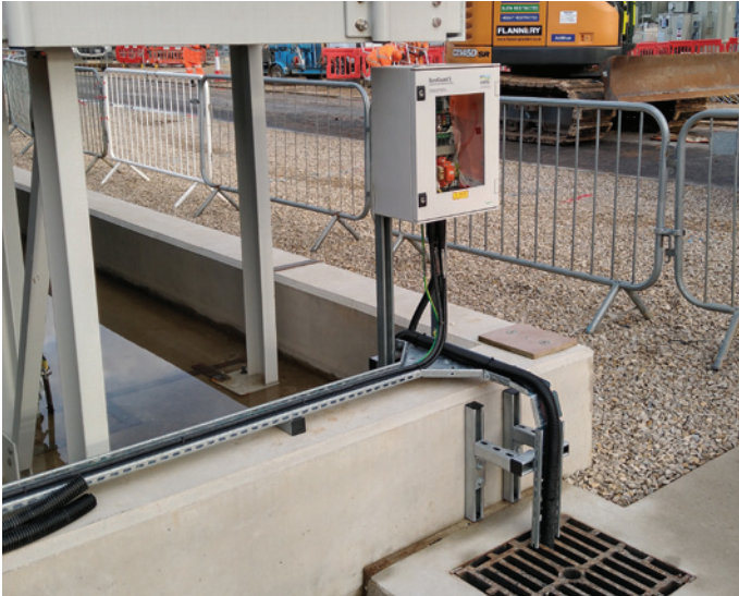
Bespoke installation using National Grid specification enclosure, designed and built with Glycol sensor system.
