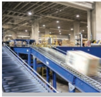
Transportation conveyor systems
