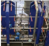
Jacking oil and seal oil systems
